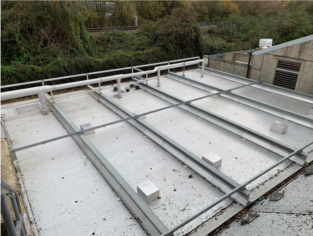
Odour control aluminium flat deck system at Portswood WWTW
