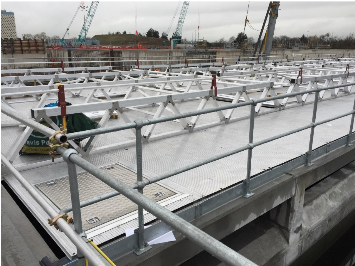
Installation of odour control aluminium flat deck system & access hatch at Deephams STW
