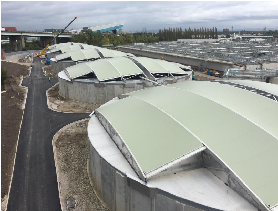
Odour control cover & aluminium flat deck system installed at Davyhulme WWTW
